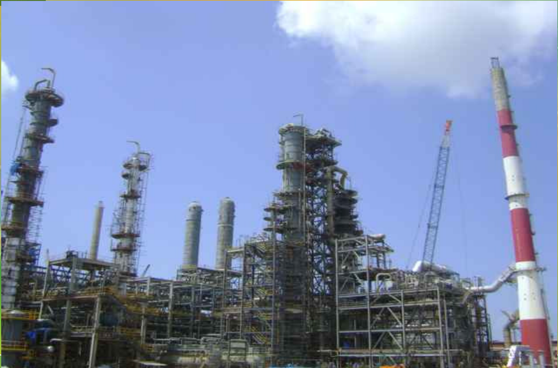
Mangalore Refinery and Petrochemicals Limited
