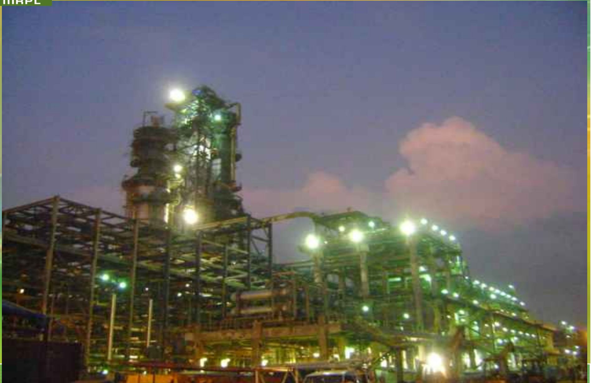
Mangalore Refinery and Petrochemicals Limited
